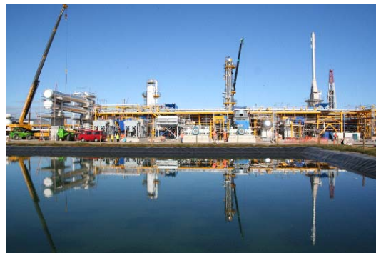
Pohokura fire water pond
