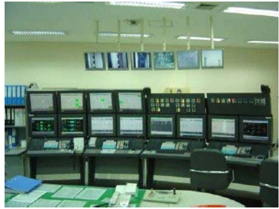
The SKC PO/SM facility uses Experion PKS technology for automation, process and quality control.
