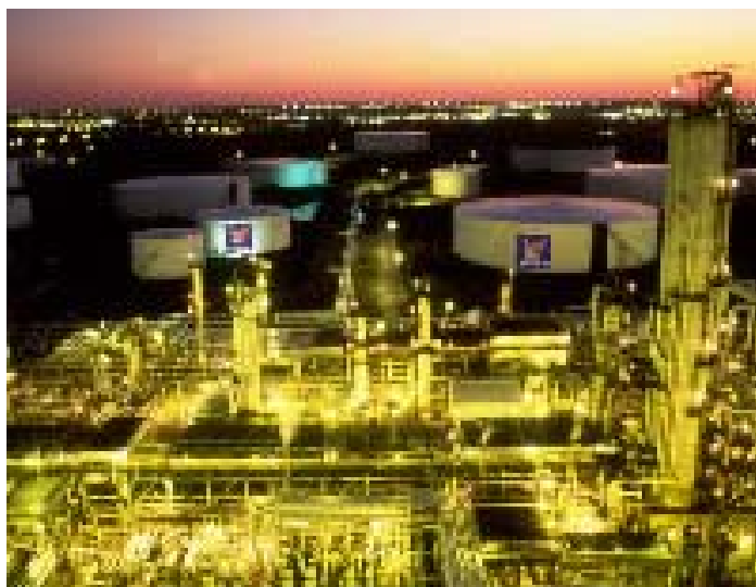
The Jean-Gaulin Refinery near Quebec City uses state-of-the-art technology for crude oil processing of 215,000 barrels per day.
