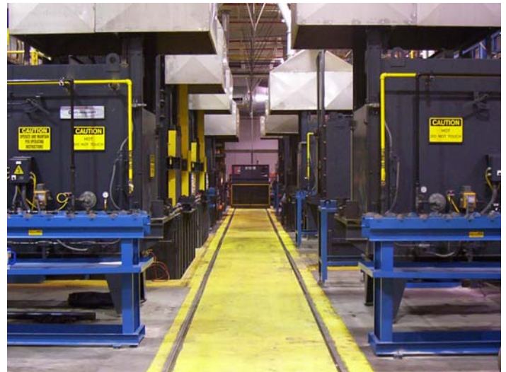
Bodycote’s heating plant uses Honeywell wireless technology to obtain needed information to monitor gas consumption
