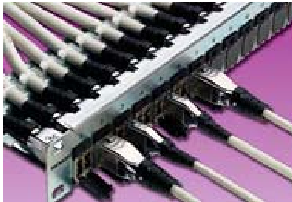
Figure 2 - Typical Screened Patch Panel (Image courtesy of The Siemon Company)
