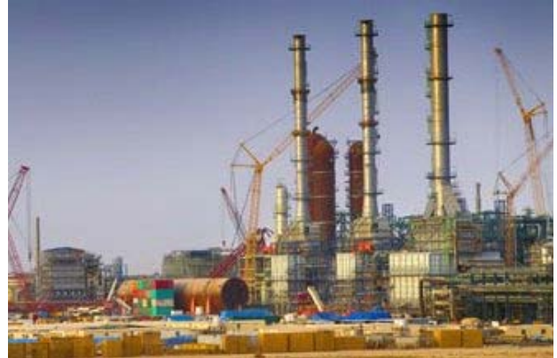
Sasol relied on Honeywell's Profit Loop to reduce energy costs at its naphtha hydrotreater in Secunda.
