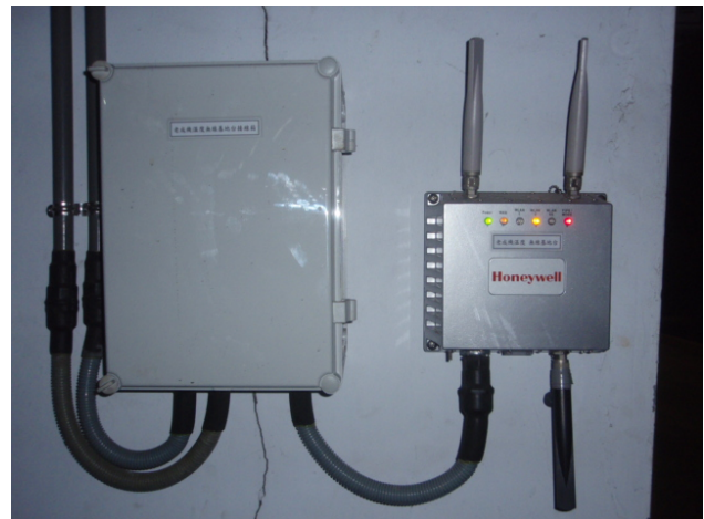
Formosa implemented Honeywell's One Wireless solution for improved process measurement.
