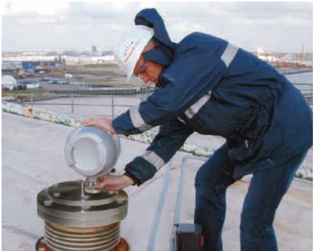
Honeywell Enraf SmartRadar wireless level gauge installed at Standic terminal, Dordrecht
