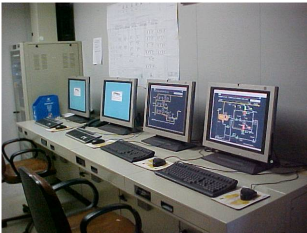
Figure 1. HMI migration is one of the most important aspects of control system modernization.
