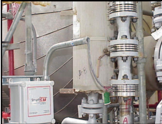
Figure 3. The SmartCET instrument, such as this one installed at a chemical plant, uses a number of electrochemical techniques for monitoring. Corrosion probes are a flow-through design installed via standard ANSI flanges.
