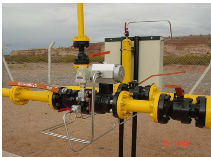
Honeywell wireless transmitters monitor pressure transmitter WG514 in fuel gas pipeline.
