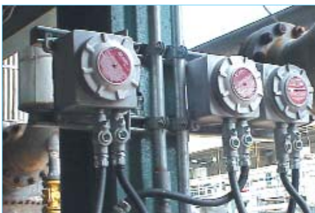
Figure 4. SmartCET corrosion analysers mounted in explosion proof enclosures.
